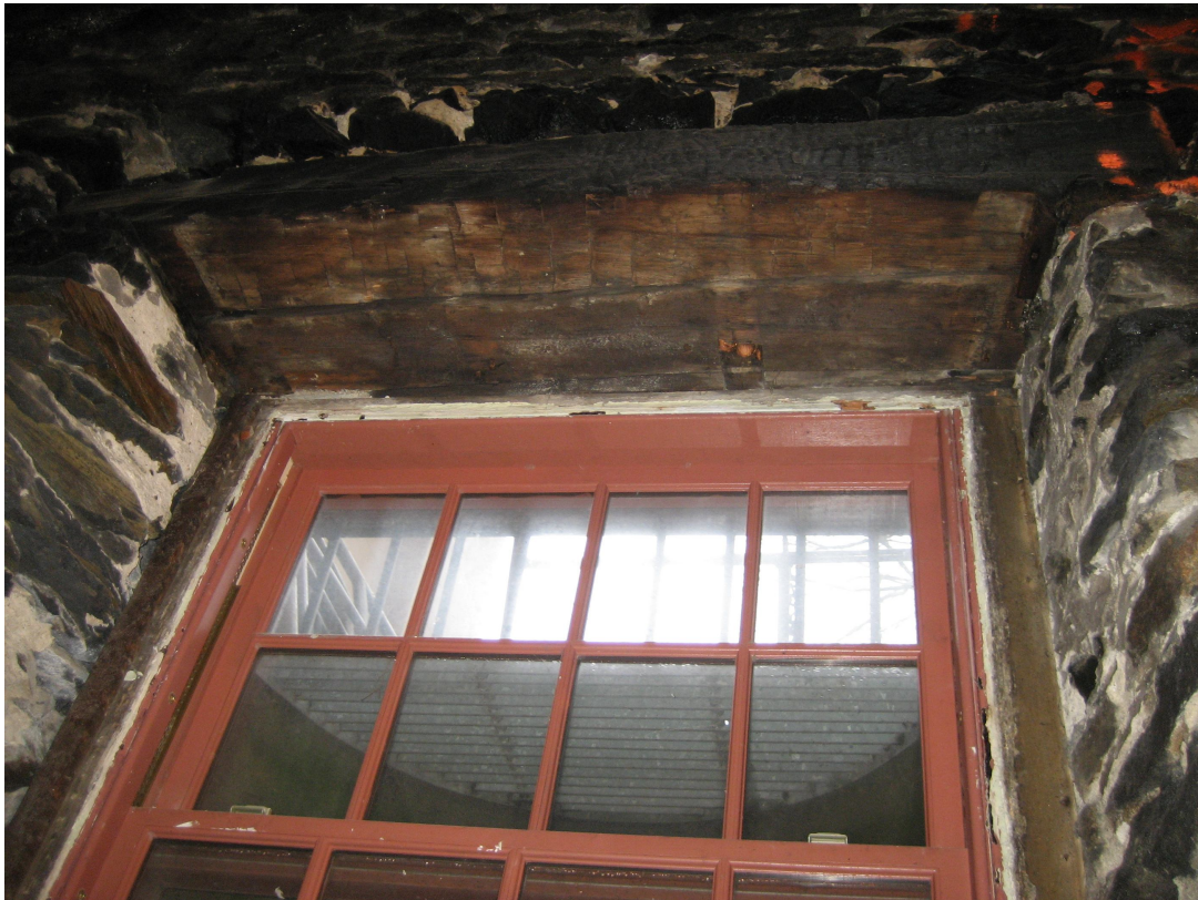
Figure 8. View of the wooden beams above the window supporting the casement in addition to a visual of the ground surface to the exterior of the building.
