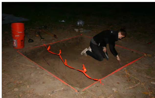
Figure 11: Excavators marked off the southern portion of the unit in order to avoid the pipe.
