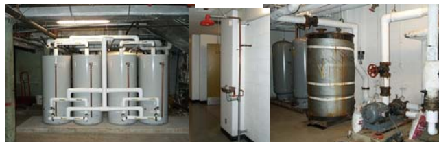
Division 2 —Installation of new domestic hot water storage tanks and pad in Caswell; and in Barus and Holley an eye wash station and two pressurized vessels and re-piping of the booster pumps.
